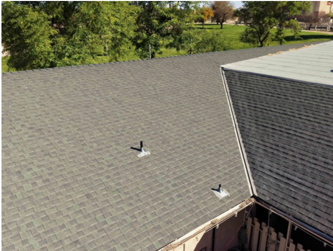
Compromised valley/edge detail. Total removal ensures we can install new ice and water shields for maximum leak protection.
