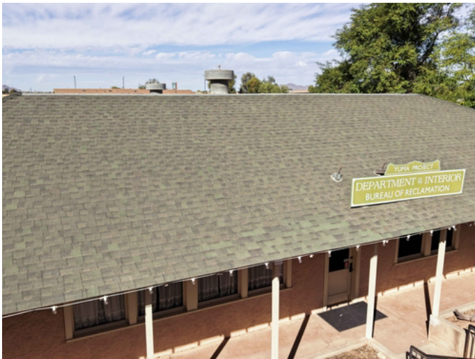
Current roofing system has surpassed its life expectancy. A full tear-off is required to inspect the underlying wood deck.
