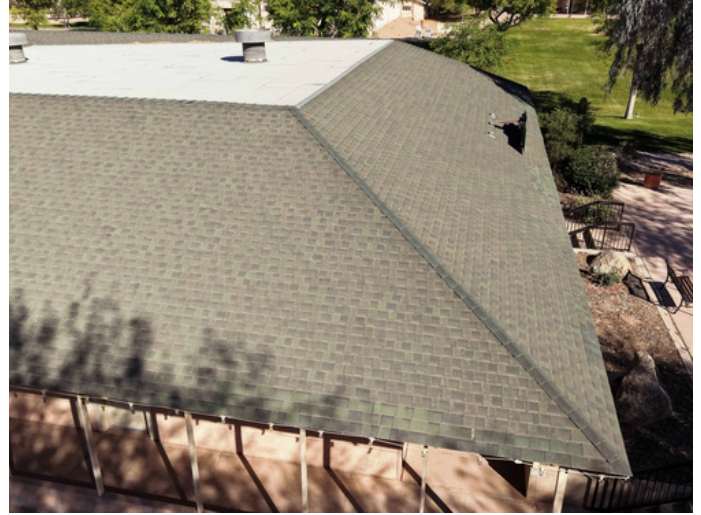
Evidence of shingle 'balding.' Without the protective granule layer, the asphalt core is exposed to UV damage, necessitating a full tear-off.
