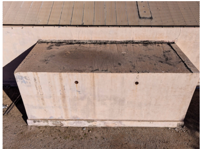
This negative pitch is causing water to pool against the building envelope, resulting in active interior leaks and moisture intrusion.
