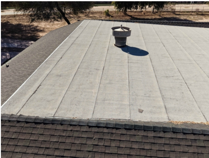
This area will be cleaned and primed to receive polyester fabric, eliminating the seams where most flat roof leaks begin
