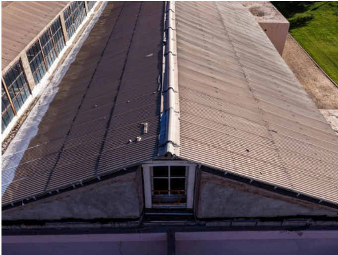
The existing ridge caps have become brittle and cracked, leaving the most vulnerable part of the roof exposed to water intrusion.
