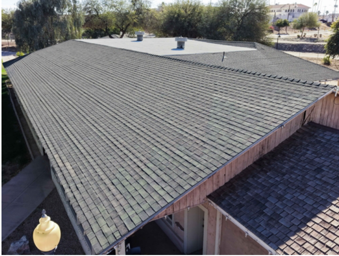
Overview of aging roof area. Visible signs of wear suggest a high risk for future leaks if not addressed with a complete replacement.
