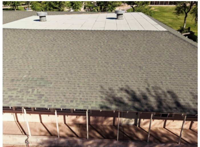
Significant thermal cracking and shingle curling. These defects allow wind-driven rain to bypass the primary drainage layer.
