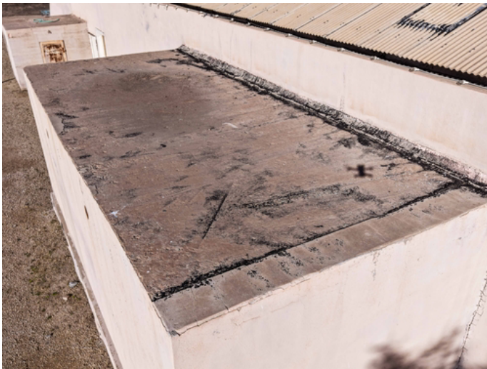
The existing concrete roof deck is sloping toward the building structure rather than the designated drainage points
