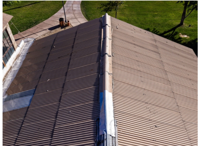
Immediate replacement with a reinforced metal ridge system is required to prevent structural damage to the ridge beam.
