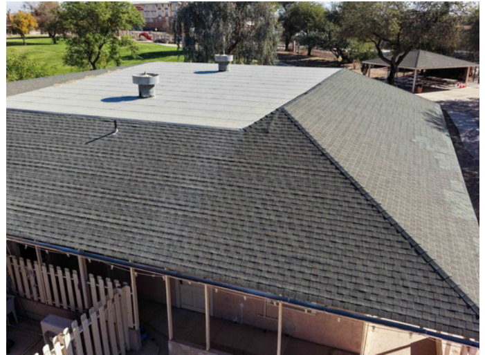
Poorly sealed penetrations and worn shingles. The new installation will include all-new flashing and high-performance underlayment.
