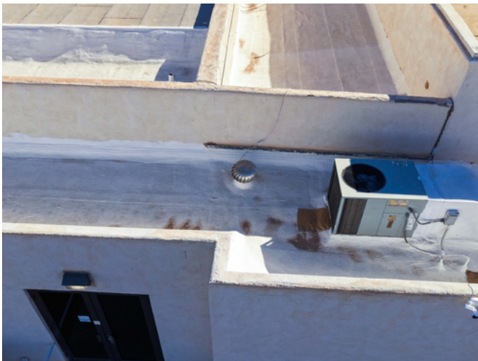
Secondary pack unit: To be removed by AC team for sub-unit sealing and waterproofing.
