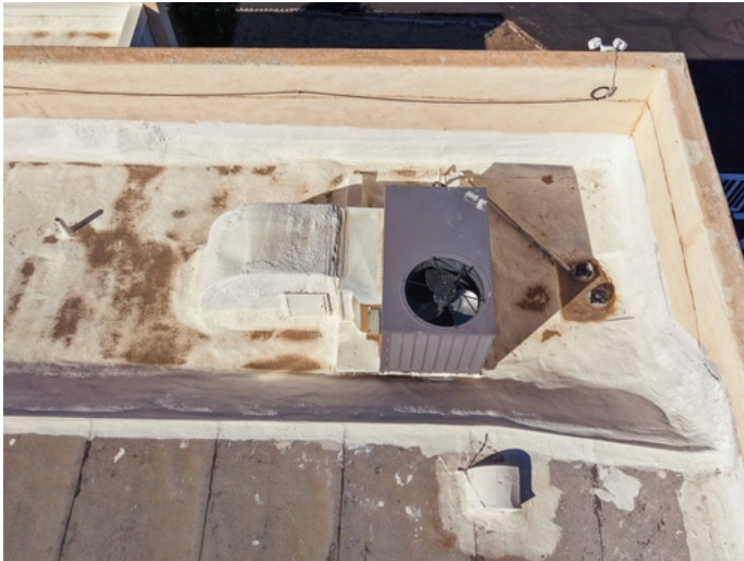
The third pack unit will be temporarily removed, allowing for the application of a reinforced coating to the underlying substrate."
