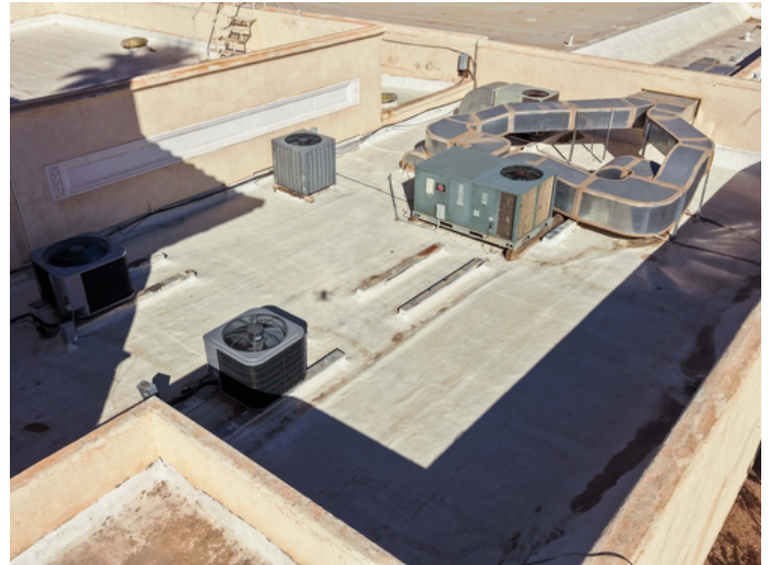
Scope includes the removal of rooftop AC units by our mechanical team. This ensures the new seal is applied to the entirety of the substrate, including beneath the units, followed by professional re-installation
