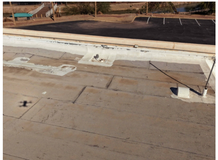
Area of failing patches, to be reinforced with polyester stitch-bonded fabric and elastomeric topcoat for maximum durability."
