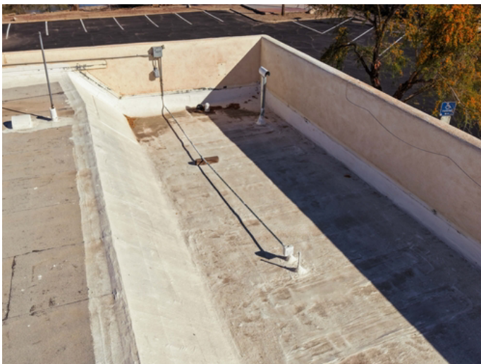
Clear all rooftop debris and perform a full-scale pressure wash to strip away chalking from the existing faded coating.
