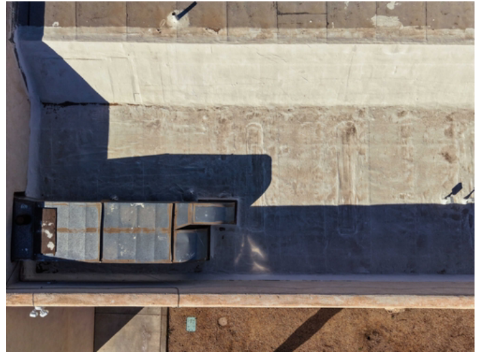
A high-pressure thermal wash will be performed to remove all chalking, debris, and atmospheric contaminants, ensuring a profiled substrate for maximum elastomeric bond strength.
