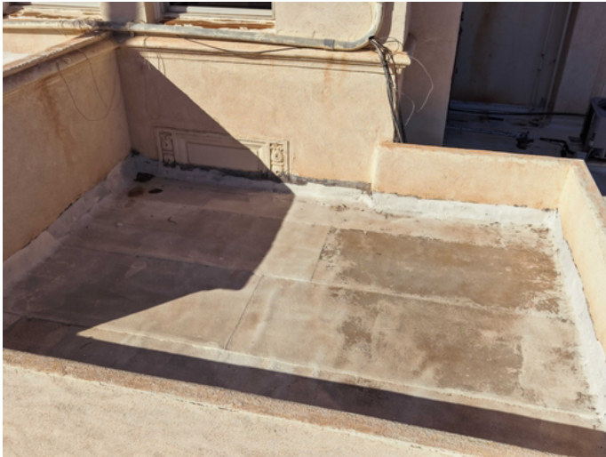
The roof displays typical wear and tear, including a fading topcoat that may no longer provide an optimal moisture barrier.
