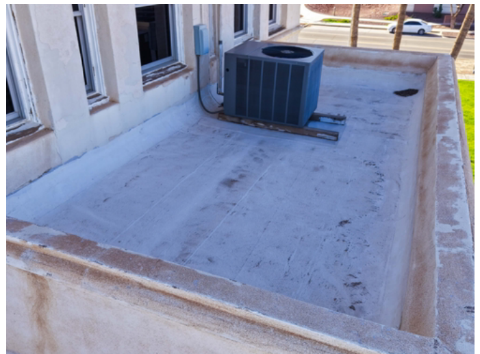
Apply protective elastomeric membrane to the entire roof surface, including all reinforced patch areas.
