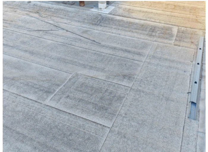
Thorough pressure washing of the entire roof area to remove all contaminants and ensure a high-strength bond for the new coating.
