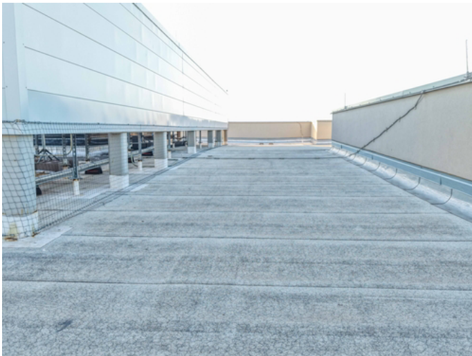
A proactive restoration system is advised to address current wear and provide long-term waterproofing.
