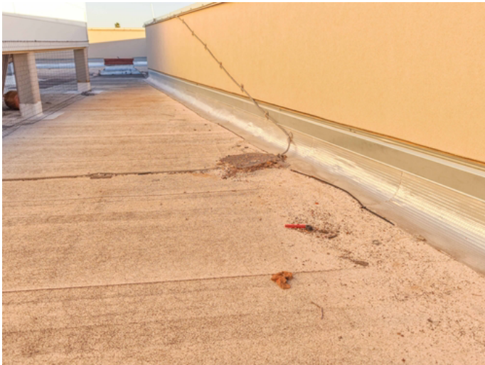
Removal of all loose debris is required to ensure proper adhesion of the new restoration system.
