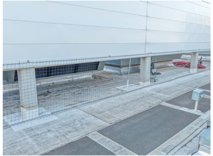
All parapet walls will be sealed up to the transition of the roofing material.
