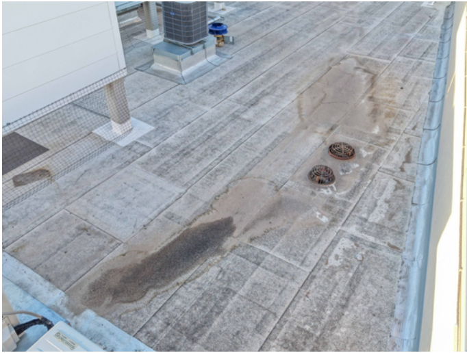
Complete clearing of all primary drains and scuppers to ensure unrestricted water flow and eliminate ponding.
