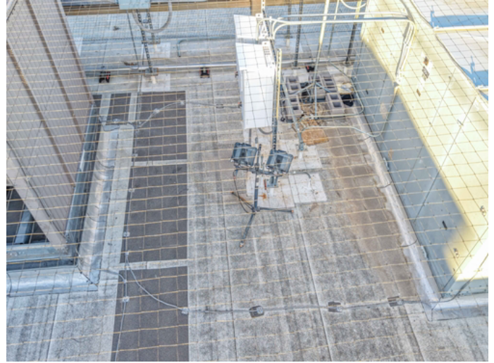
Evidence of UV degradation and membrane thinning, compromising the roof's waterproofing
