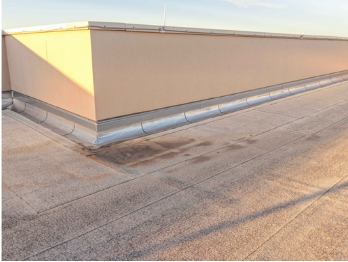
Signs of standing water; indicates inadequate drainage or deflection in the roof deck.
