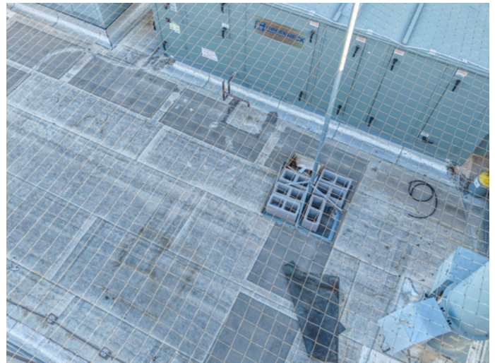
Clean and seal all mechanical unit curbs with flashing-grade sealant to prevent moisture infiltration at the base.
