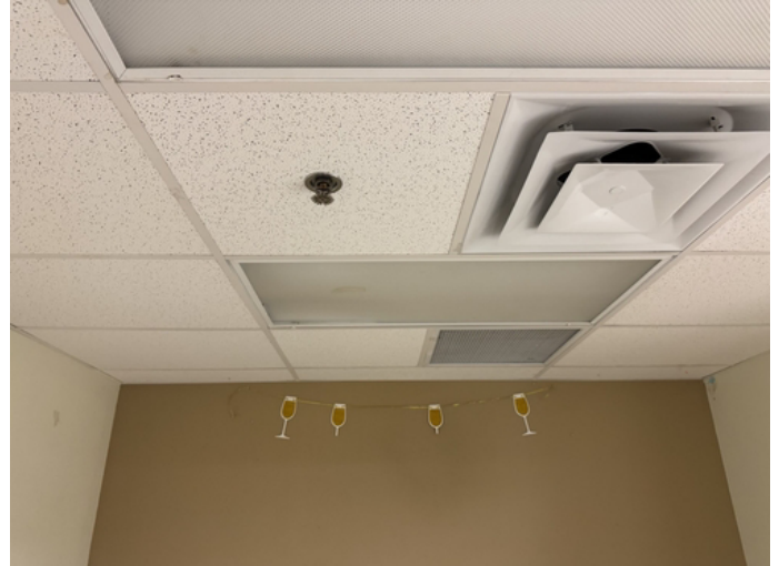
Interior tile with water stains
